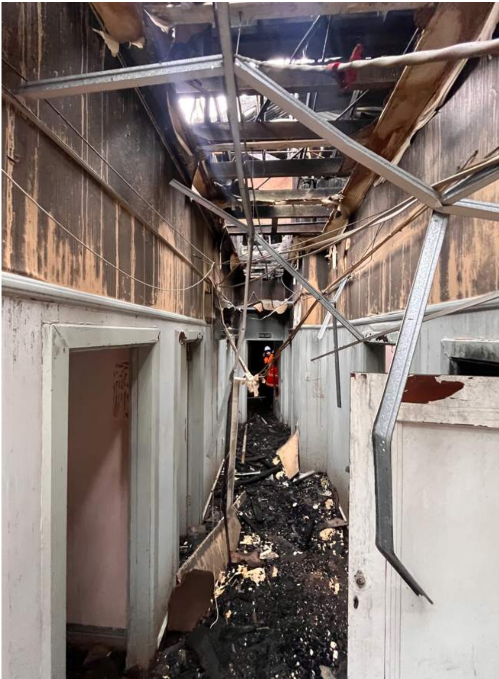
EASTERN PORTION OF THE BUILDING - FIRE & SMOKE DAMAGED
