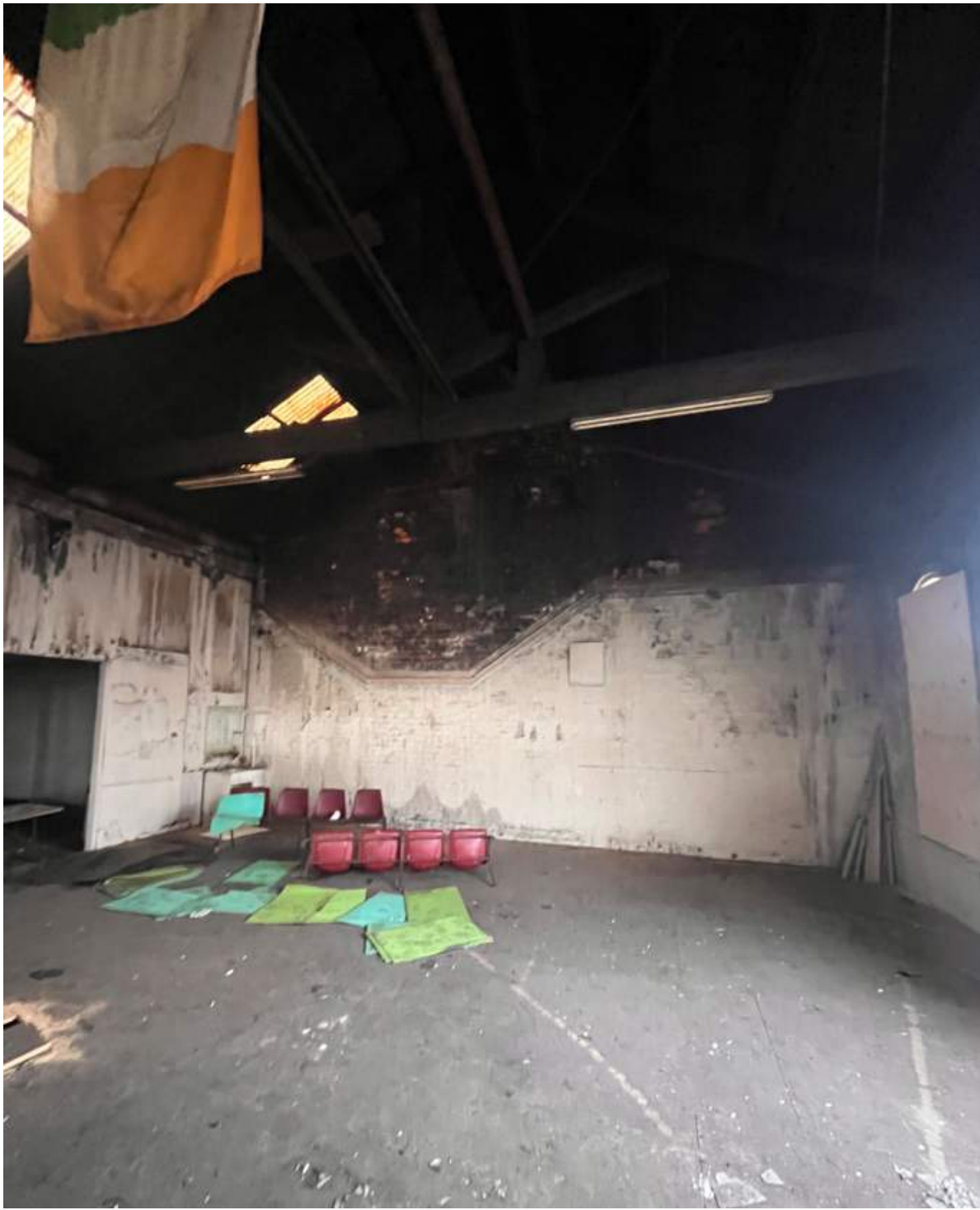
WESTERN PORTION OF THE BUILDING - SMOKE DAMAGED
