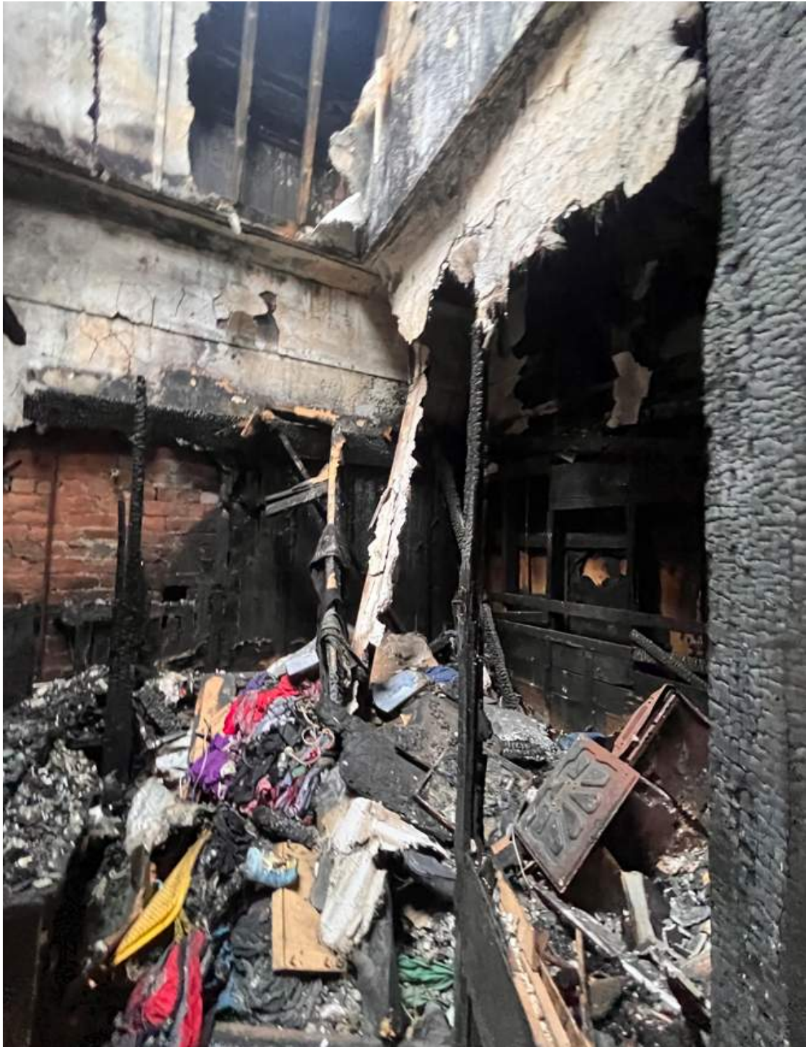
EASTERN PORTION OF THE BUILDING - FIRE & SMOKE DAMAGED
