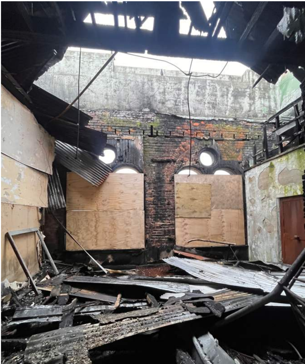
EASTERN PORTION OF THE BUILDING - FIRE & SMOKE DAMAGED
